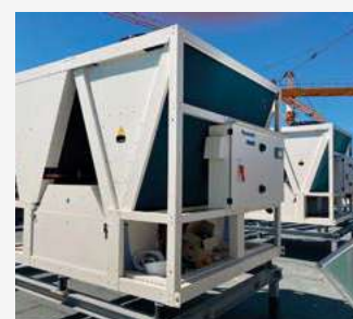
Hungarian Cédrus Liget. A complex facility including apartments, offices and commercial units. Szeged, Hungary. ECOi-W, ECOi and ERV.
