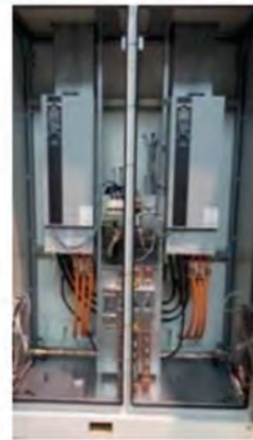
Compressor drives + main power connection
